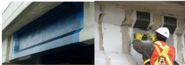
Figure. 3. Strengthening of RC girder by CFRP laminates in shear (M.B.S Alferjani et al 2013).
