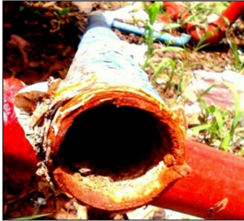
Fig 2. Internal corrosion in piping's:
