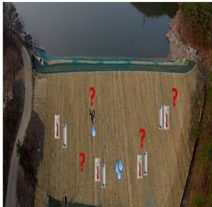
Figure 3.1 Site View of Anomaly occurrence taken by Drone
