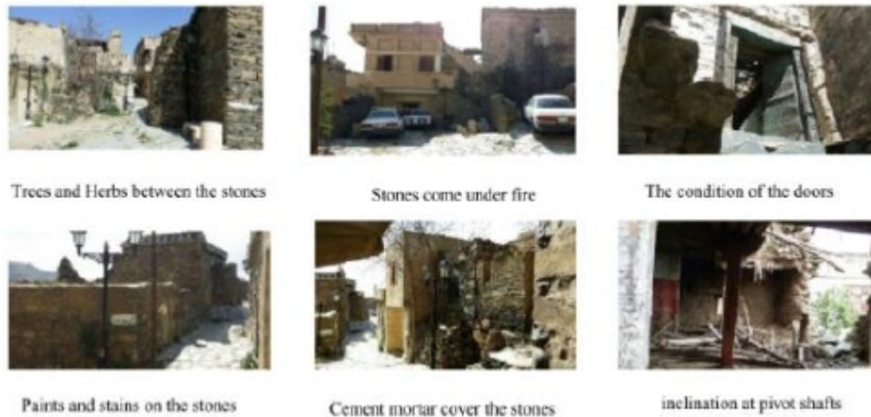
figure 12: the problems that have been detected in the stones of the village Source: researcher
