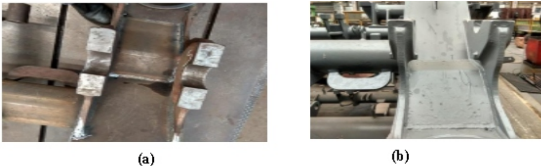
Fig.5 (a) Gap between control arms and (b) Gap between control arms after rectification
